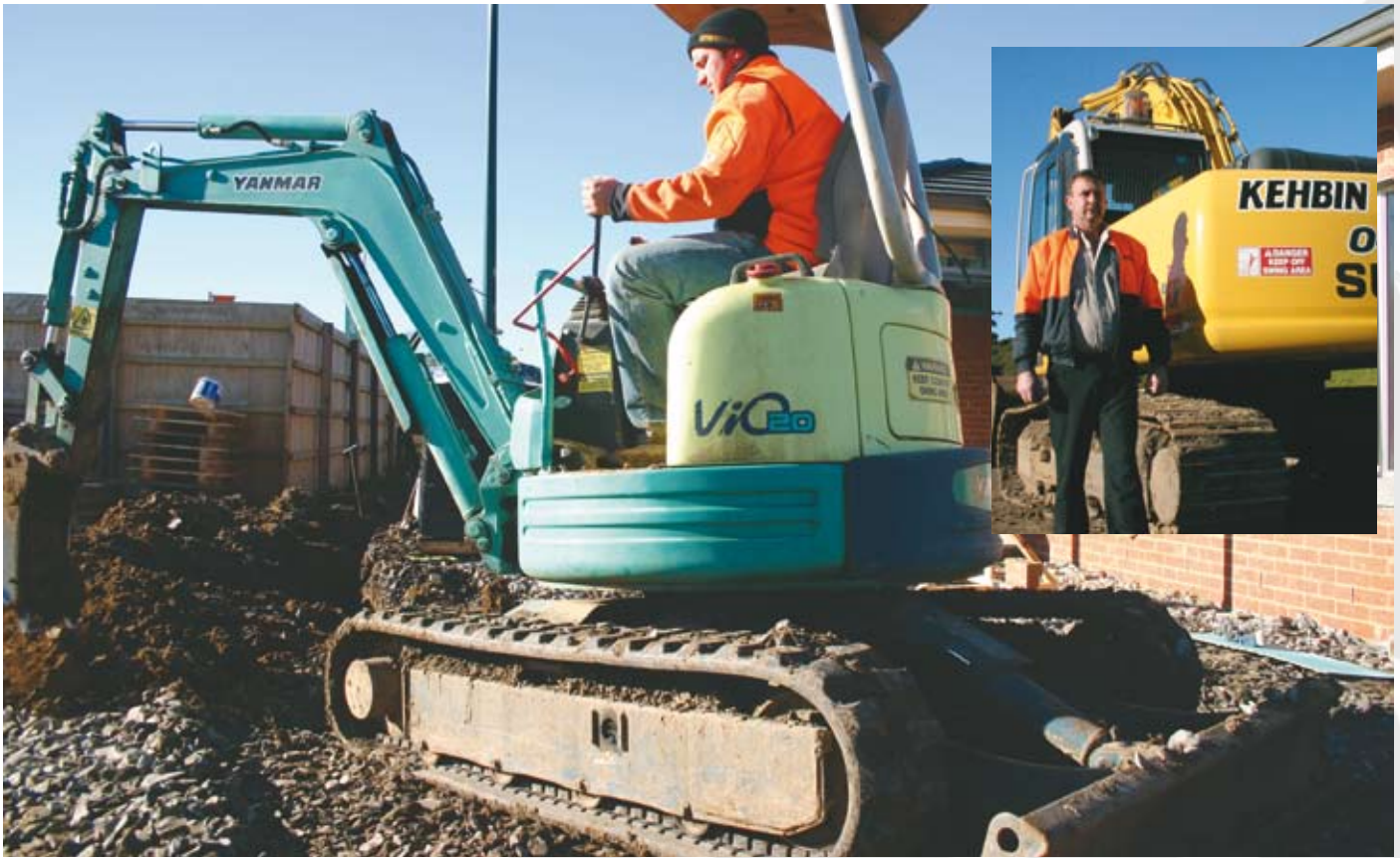
Kehbin's 2 tonne mini excavator, fitted with Bridgestone rubber tracks. Inset, Wayne Francis, owner of Kehbin Pty Ltd.
